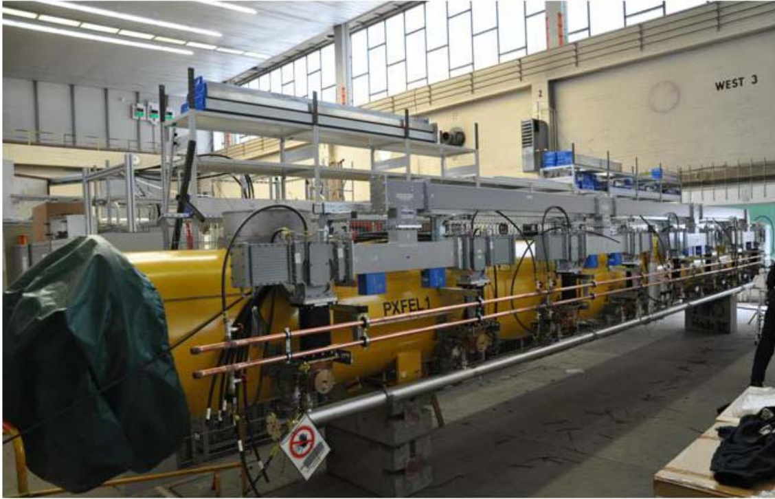
Fig. 5: Accelerator module and RF waveguide distribution
