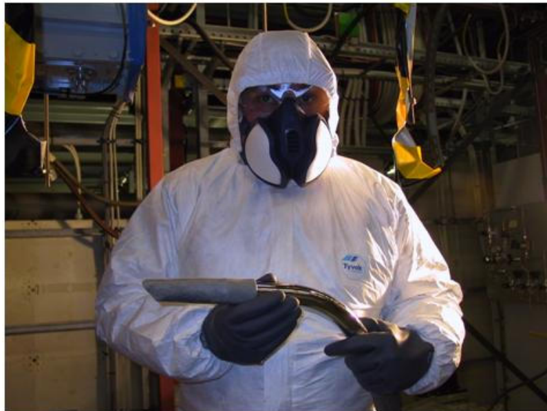
Fig. 9: Staff wearing protection clothes during work at \text{SF}_6 waveguides
