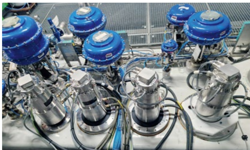
Figure 1: Cold compressor motors with active magnetic bearings (metallic pillars in the front) installed in the 2 K cold box
