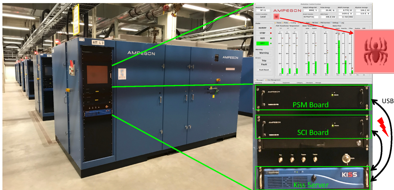
Figure 1: High voltage modulator, GUI and control system.
