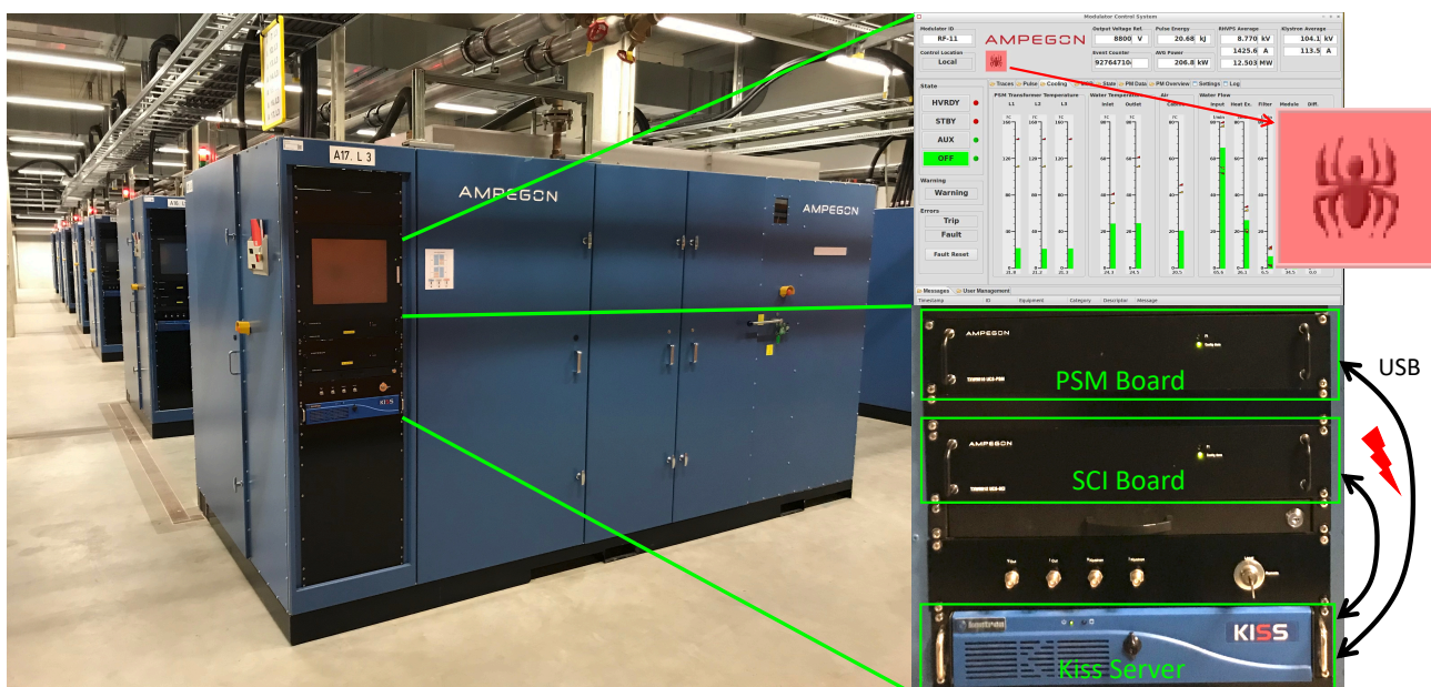
Figure 1: High voltage modulator, GUI and control system.
