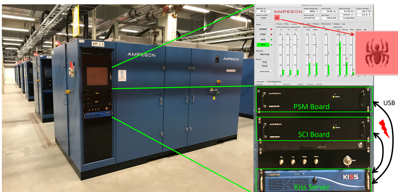
Figure 1: High voltage modulator, GUI and control system.
