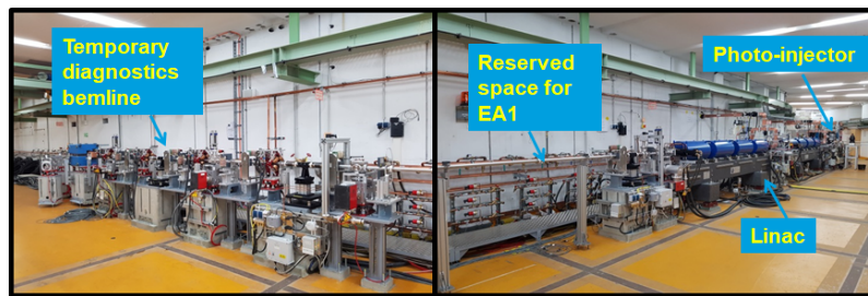
Figure 2. Present status of the installation of ARES. The pictures are taken from the middle of the tunnel looking on the left and right side respectively. The layout shown corresponds to the one on top of Fig. 1 but the experimental area EA1 has not been installed yet (a straight vacuum pipe reserves the area).
