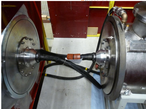
HV cable #1, leakage current ~ 2A
