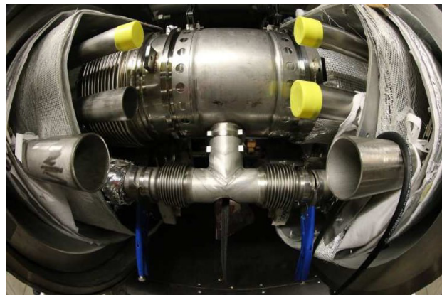
Figure 13: A typical module-module connection, where only the gas return pipe and 2-phase line are positioned for the first weld operations.
